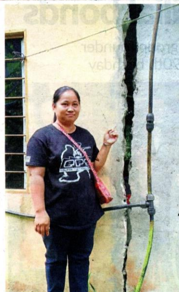
Surayati showing the massive crack on a wall of her home.
